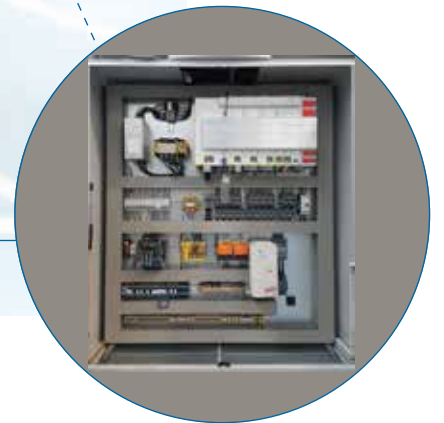
EASY ACCESS TO THE ELECTRICAL CABINET
